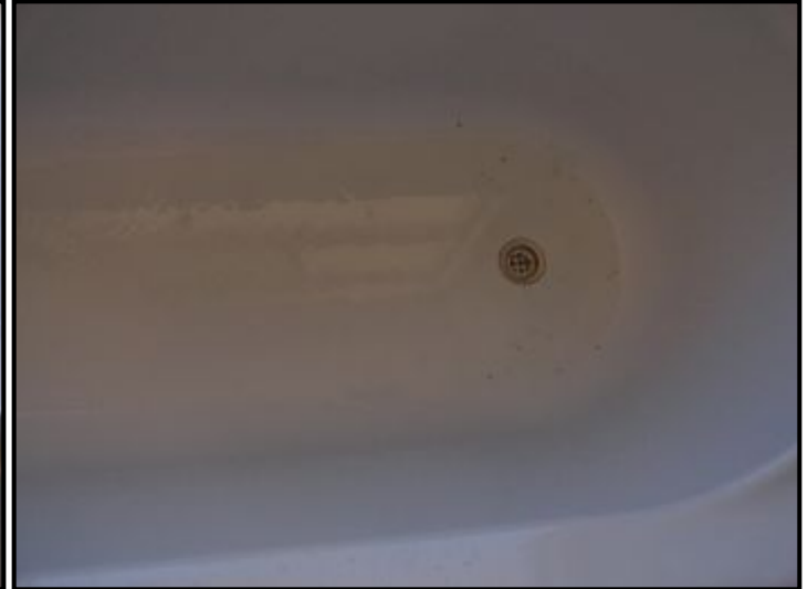
Noted that bath tub drained slowly.
