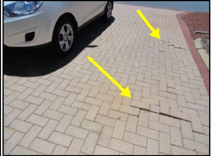
Uneven pavers noted to some areas.
