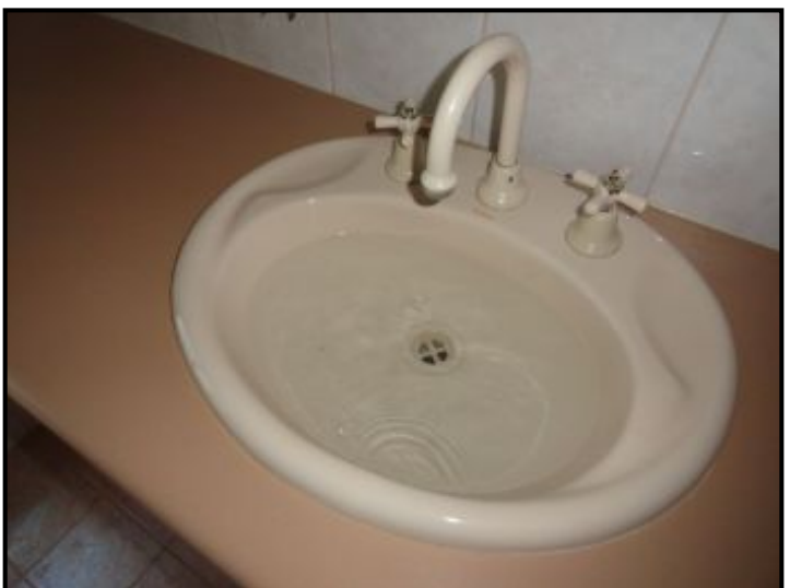
The sink in the en suite bathroom drained slowly.
