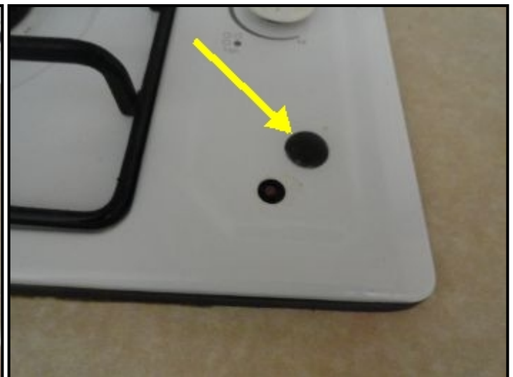
Noted that ignitor button was loose
