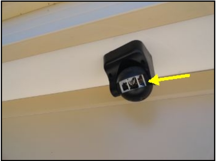
Damaged light sensor noted
