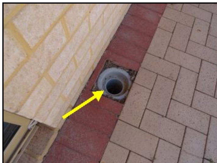
Drain pipe missing a grate.
