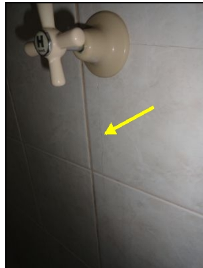
Cracked tiles noted
