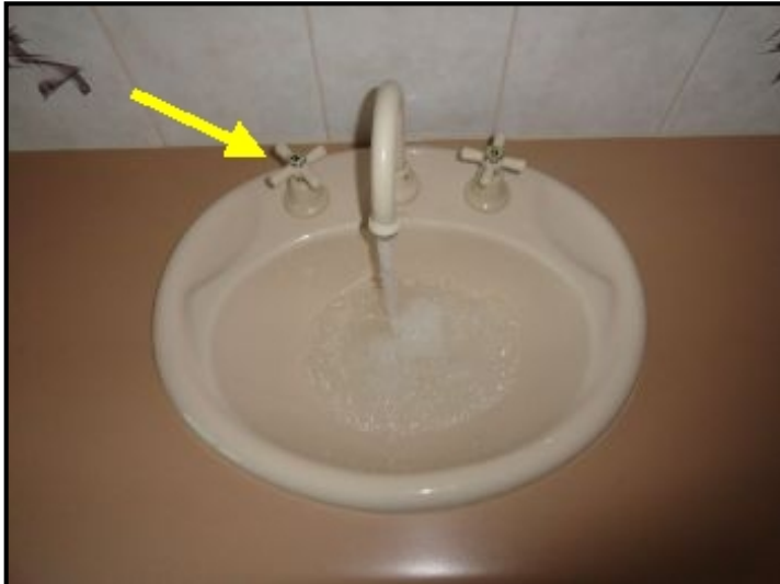
Taps were stiff to operate
