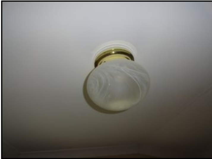
Bathroom Light did not work
